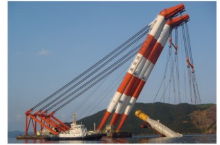
3. The floating body is lifted and raised by a large floating crane, and floated on the sea.
