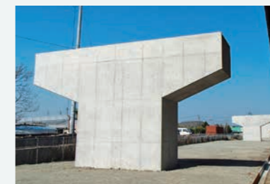
Yamoto Ishinomaki Highway substructure construction Tohoku Regional Development Bureau, Ministry of Land, Infrastructure, Transport and Tourism
